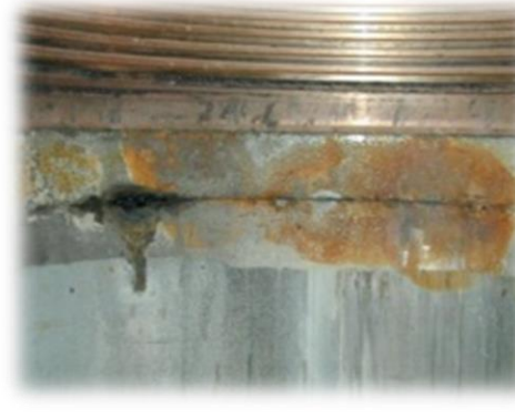
Crevice Corrosion (narrow Clearances)
